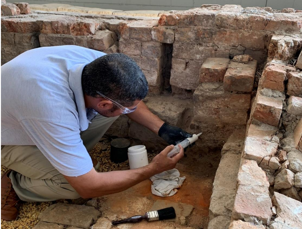
Plate 10: Early convict settlement at V by Crown, Parramatta – showing repair of wasp burrows
