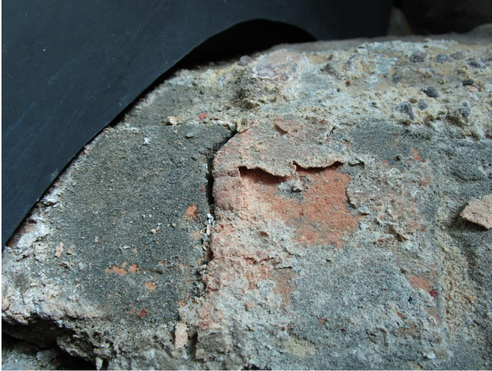
Plate 14: First Government House at Museum of Sydney –showing development of salt efflorescence 'crust' and associated damage from detachment
