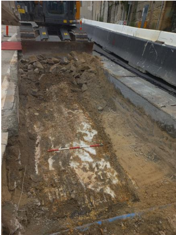
Figure 4.17: Cut-down sandstone bedrock as found immediately beneath the road construction fills in Trench 2.2. View to the north. Scale 1m.
