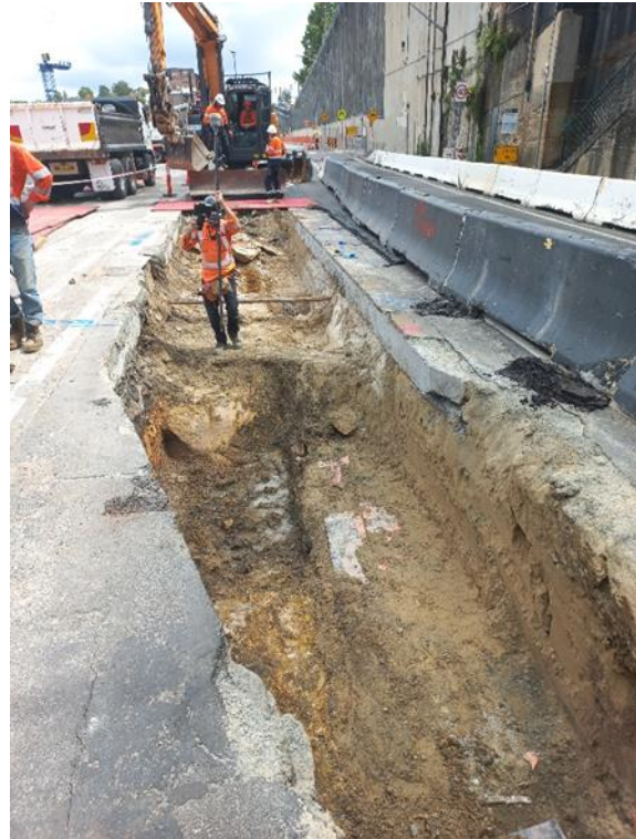
Figure 4.18: Looking north along Trench 2.2 showing the deep service trench on the right and the small dark brown patch of clay fill (016) in the foreground.
