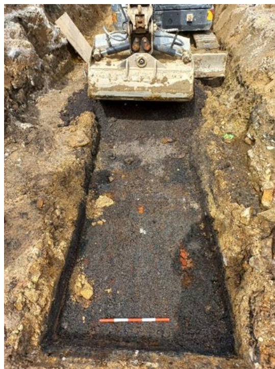
Figure 4.23: The sandstone rubble was capped with a fill of loose, coarse industrial waste. Scale 500mm. view to the southwest.
