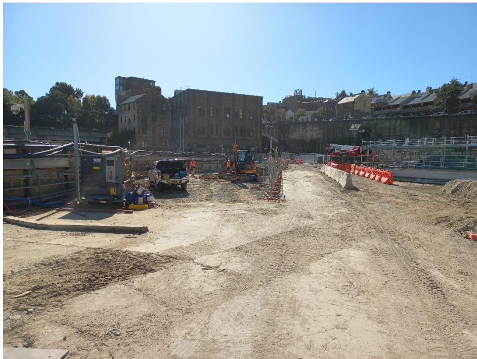
Figure 4.35: Area of excavation (left) looking north with the Dalgety Bond Store (25 Hickson Road) beyond, and the Hickson Road retaining wall and cutting at the right.
