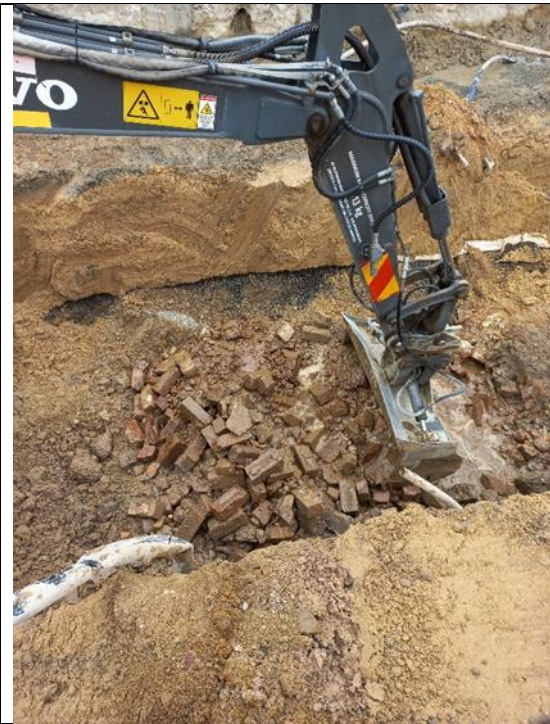
Figure 4.31: Sand and modern construction material dominated the bulk fills in the stormwater trench. The clean sand and gravel fill of deep services can be seen on the far (eastern) side of the trench. View to the east at the southern end of the stormwater excavation
