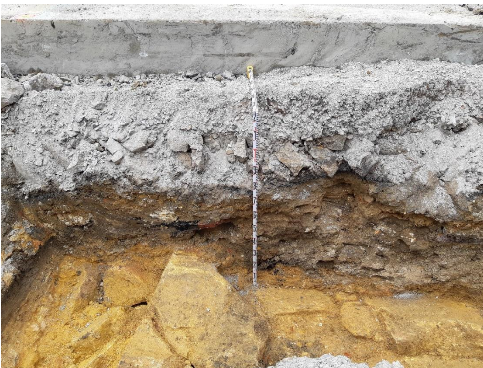
Figure 4.13: Sandstone rubble used as base reclamation fill (012) shown immediately beneath the clay construction fills for the road. All significant archaeology was removed from this area.
