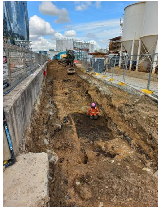
Figure 4.32: Only a small patch of archaeology (seen here as dark soil) was preserved in the stormwater trench. View to the southwest
