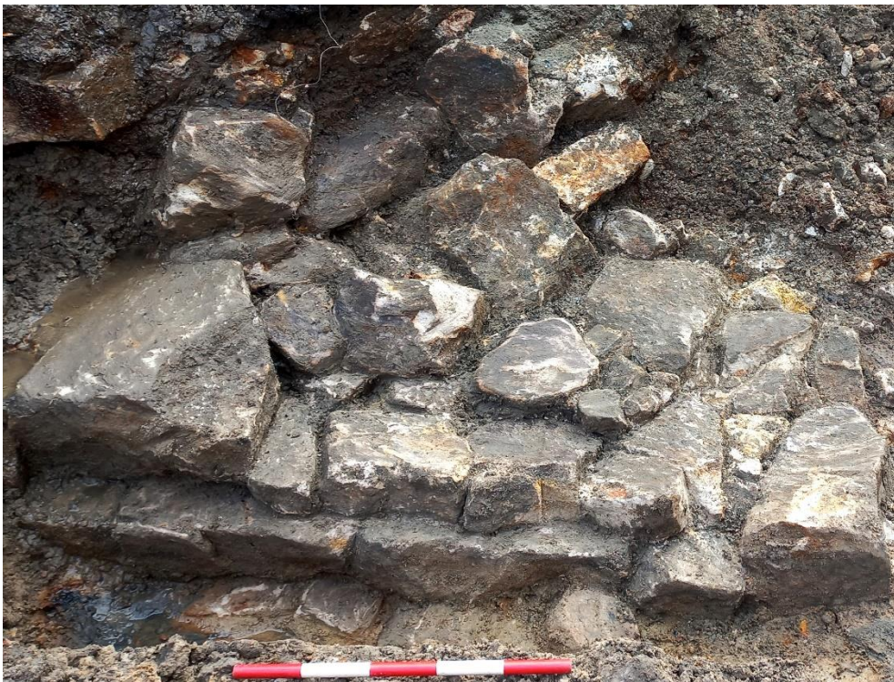
Figure 4.59: Exterior face of the wall showing considerable damage to the upper course. Scale 1m. View to the north.
