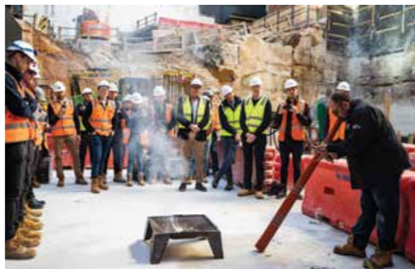
Indigenous smoking ceremony at a BESIX Watpac project site - held within a designated safety exclusion zone with all works ceased.
